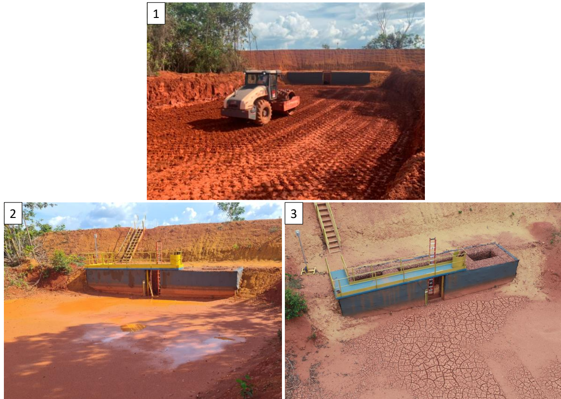
Figure 4 Compaction around the spillway (4-1), silting during the rainy season (4-2) and dry season (4-3)
